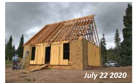
The roof was probably the most complex and most difficult portion of the building process.
