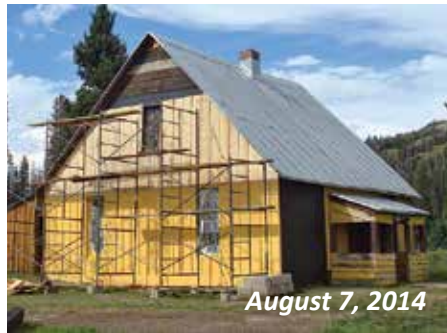
New framing and sheathing replaced the old on the Chama side of the building.
