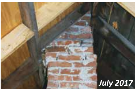
An accident waiting to happen. Unless it's repaired, one might need to wear a hard hat inside the building.
