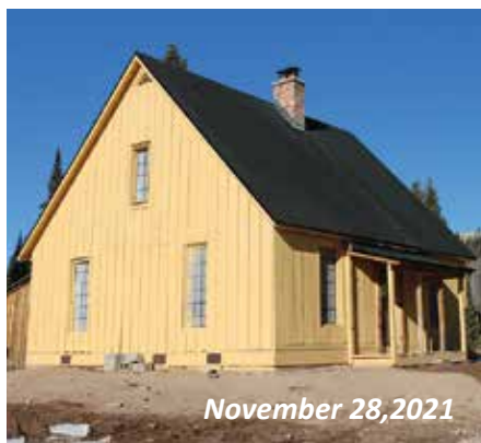
Temporary windows and doors in place and with complete final roof installation, the Car Inspector's House is ready for the winter.
