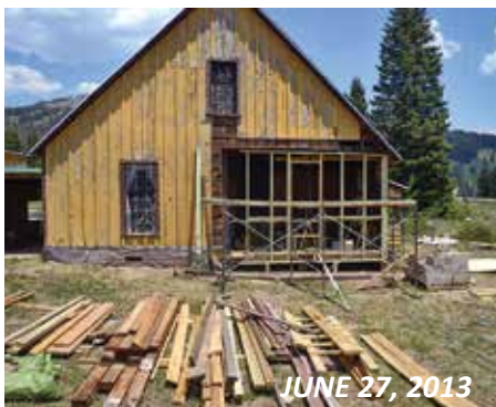
The location of the old garage door was rebuilt with stronger materials.
