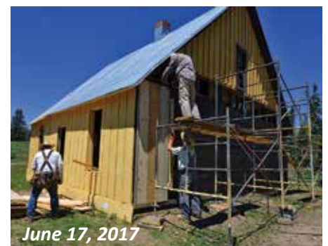
After waiting out the winter, the Antonito (north) side of the structure was also re-sheathed with board and batten siding.
