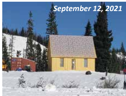
Almost completed for the season, the Car Inspector's House awaits its new, historically-accurate roof.
