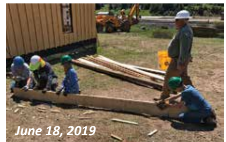
A number of young contractors, especially skilled at pulling nails, joined in including Dax Pierce, third from the left and on the far right, Clayton Buttram.
