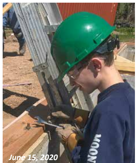
Clayton Buttram, Vance Behr's grandson, tightens the nuts on the sill plate before framing begins.
