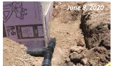
Keeping the moisture away from the foundation was paramount to the long-term stability of the entire structure.
