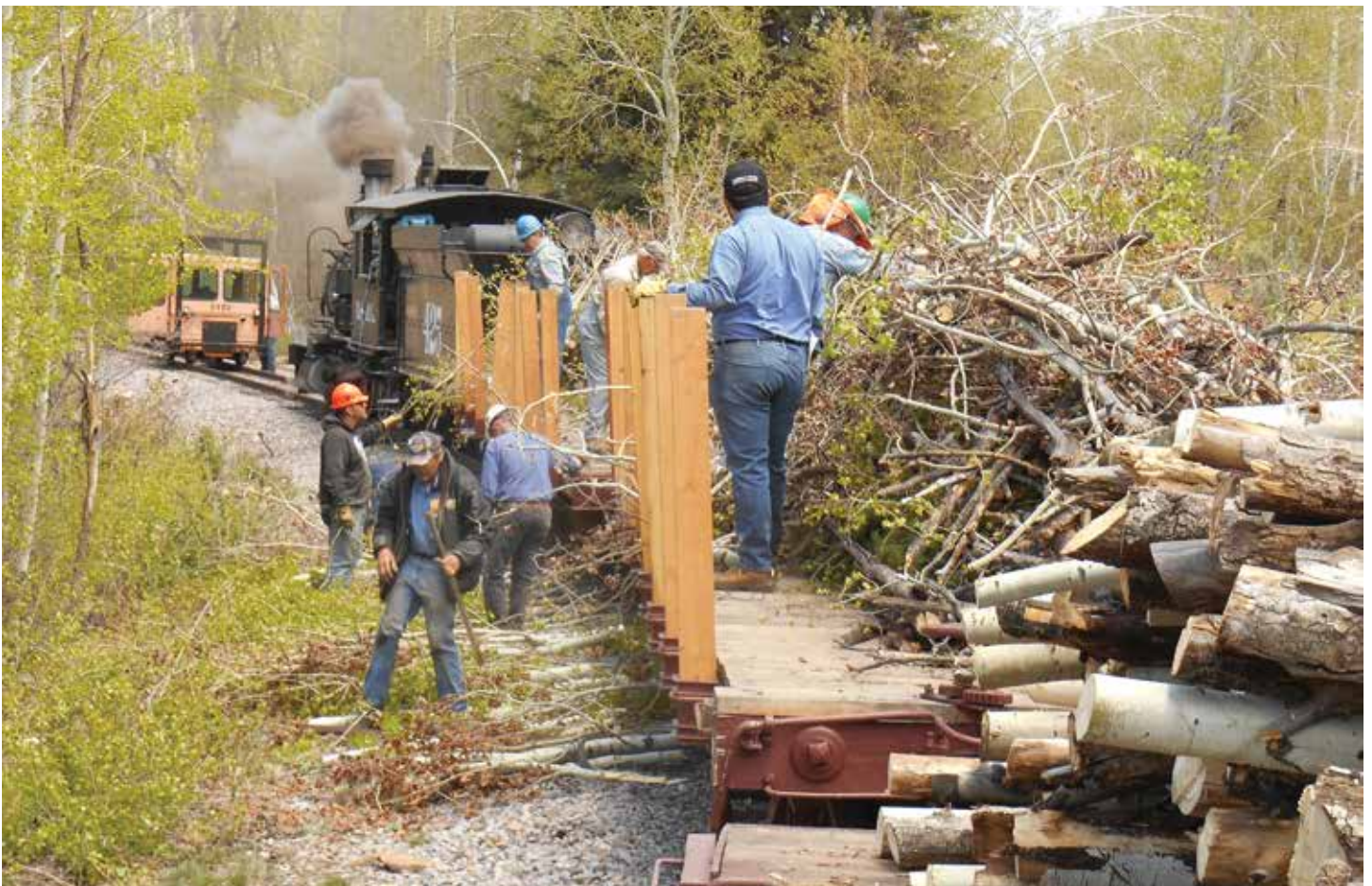
Over four days, the cutting, loading and stacking teams worked in concert to clear the vegetation in a safe and efficient manner.
