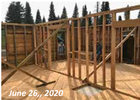
The interior load-bearing walls serve two purposes; dividing the first floor layout and providing support for the second floor joists.
