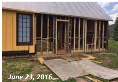
Much of the building’s front exterior was torn down to the studs for repair or replacement, then re-sheathed.
