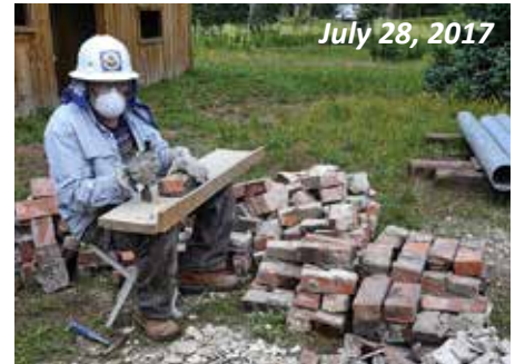
Removing the bricks was not the final step of the disassembly. George Trever cleaned and sorted the old bricks for future use.
