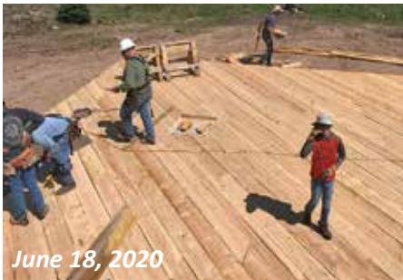
The first floor is in place, ready for the return of the saved walls. Note the location of the chimney pad.
