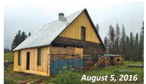
With the front sheathed in, work moved to the Antonito side of the house. Time ran out and the east wall wasn’t completed. Take note of the far end of the building and you will see a degree of “sag” in both the roof line and the bottom of the wall.
