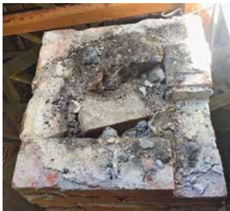
For unknown reasons bricks and debris had been used to plug the single-flue chimney.
