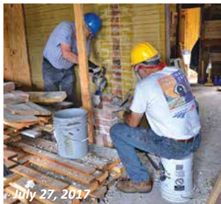
Brick by brick, the chimney was disassembled down to its base and footing.
