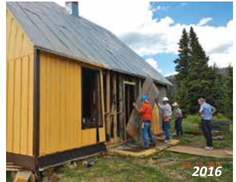
The crew begins installing the inside sheathing around the door before adding the board and batten exterior.
