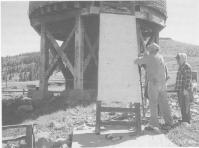
Gene Balderston, Ron Carder, and Emmanuel Lopez installing the water tank safety door.
