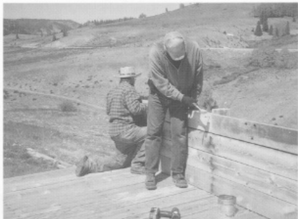
Bruce Bloom and Fuzzy Anstine installing final boards on Osier coal deck.
