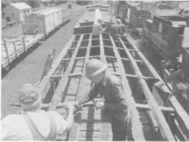
Robert Thomas, Scott Hardy, George Detwiler, and Frank Smucker have removed almost all of the roof boards on Stock Car 5549
