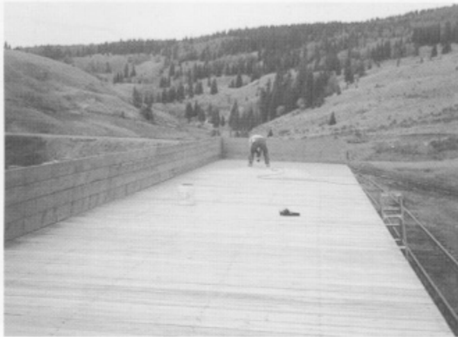
John Norcross applying grey stain to the floor of the Osier coal deck. Looks very lonely!
