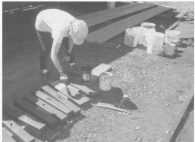
Linda King painting the final coat on the roof walk supports for car 04407.
