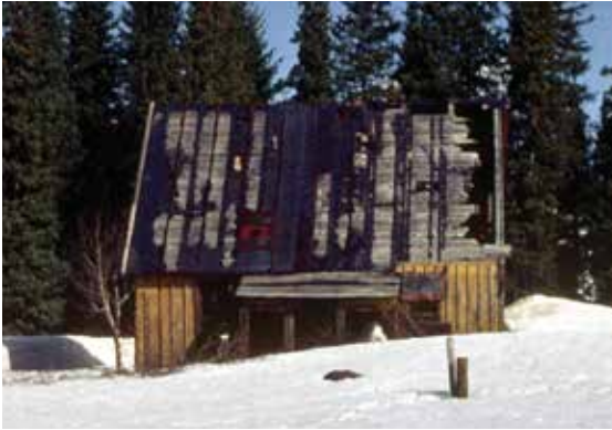
The Car Inspector's House as it appeared in the winter of 1979. The track-side-facing roof took the brunt of the sun and wind damage.
