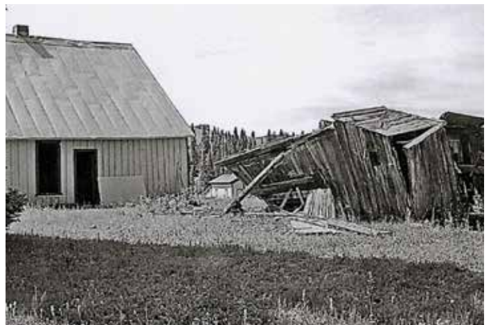
Behind the Inspector's House, the annex was basically a pile of rubble. Photo by Lynn Huber
