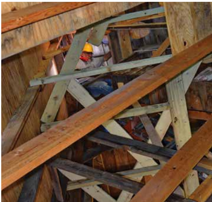
Additional structural support was added in the attic in 2008 for long-term stability as no specific plans for the Inspector's House were on the table. Photo by Friends Chronicling Team
