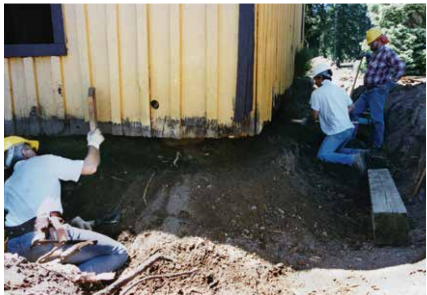
1995: Digging out the the original, rotten foundation and raising the structure to place a new, treated wood foundation and sill was arduous work. Photo by C. Edward Walton
