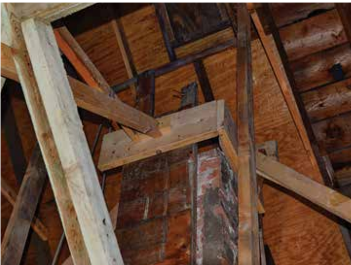
Some of the many attempts to shore up the roof rafters and rafter cross ties. Photo by Friends Chronicle Team
