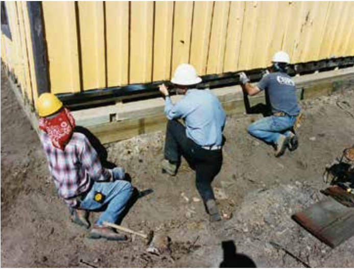
With the building raised slightly, a 10 x 10 treated wood foundation and sill plate was installed under the entire building. Photo by C. Edward Walton
