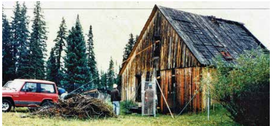
Car, plus chain, plus building? It would appear that the 1990 Friends crew is attempting to square up the sagging building so reinforcements can be placed. The building's color clearly shows the deterioration. You can see evidence of the covered-over garage door in the near corner of both of these photos.
