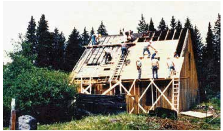
Initial roof repairs were begun in 1990 with at least ten Friends removing the old roofing material and replacing it with new sheathing. Photo by Tina Tebbens
