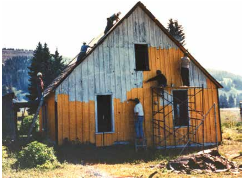
With work ongoing up on the roof, a Friends crew begins painting the Chama side of the structure. Photo by Tina Tebbens
