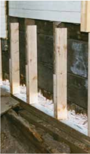
New sistered studs are attached to the new sill plate and original studs. Photo by C. Edward Walton
