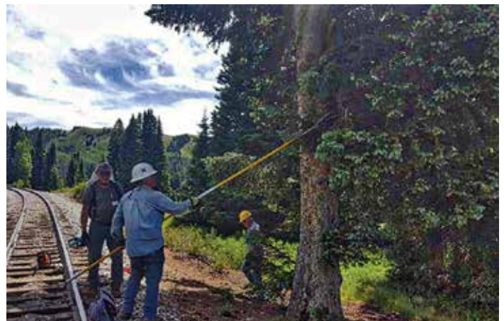
With a pole saw, the crew creates adequate set-back of the branches, not only to lessen the risk of fire but also to keep the branches out of reach of curious passengers. Photo: Ron Hassell
