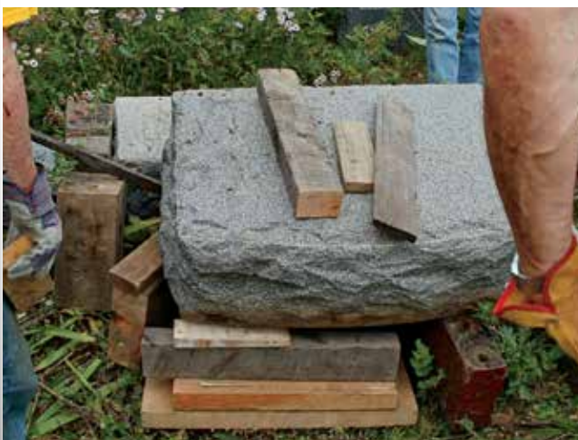
First, the 400-600 pound block of granite had to be raised with pry bars and timbers to the level of the base.
