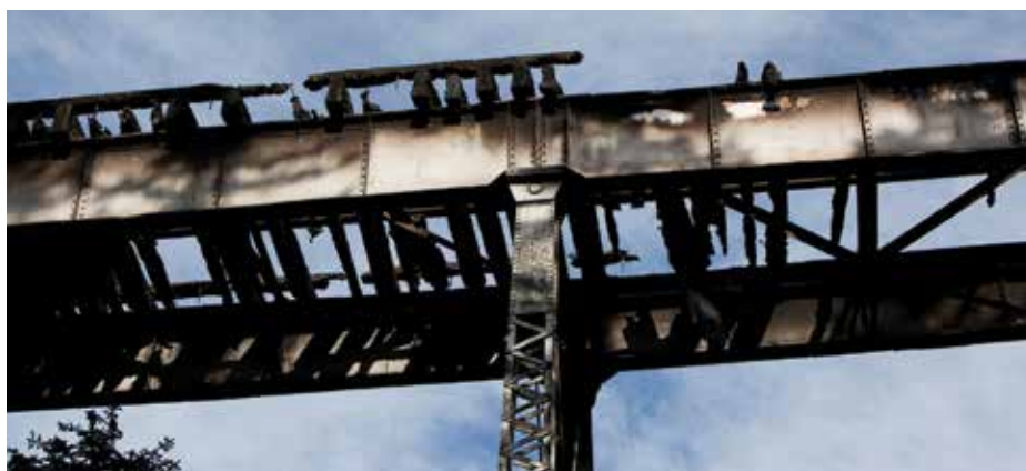
The damage, as seen from below
