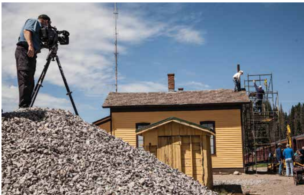
Rob Van Camp trains his lens on Bob Conry and crew as they install the new semaphore pole on the Cumbres Pass Section House.
