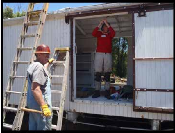
TL Craig McMullen waits for Patricia Sandt to finish tightening a bolt inside the car
