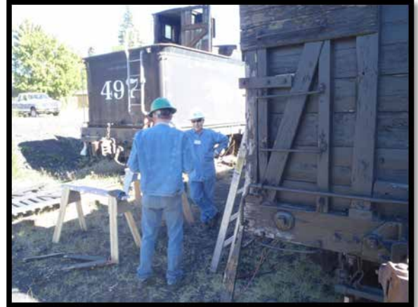
TL Scott Hardy discusses work being done on the stock cars with Site Leader Bob Craine
