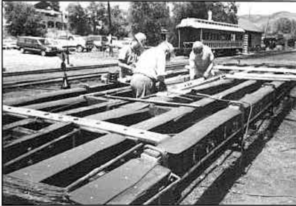
Working on the new floor for a flat car at Chama. In the background a crew from Hollywood is remodeling the Hinman coach for "The Legend of Wyatt Earp." August 1993. Photograph by Art Nichols.
