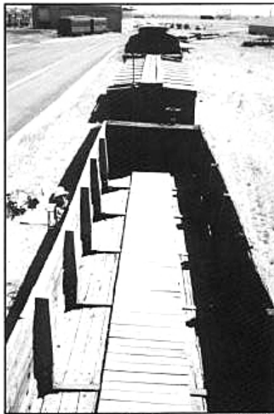
New flooring and side stakes were installed in the display train gondola at Antonito. July 1993. Photograph by Art Nichols.
