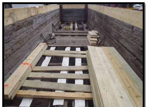
The rotted floor lumber has been removed and rubber membrane strips have been placed over the sills to repel water
