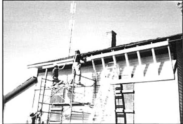
Installing temporary knee braces on the east side of the section house at Cumbres to support the roof and eaves, which were collapsing because of the winter snow load. August 1993. Photograph by Art Nichols.
