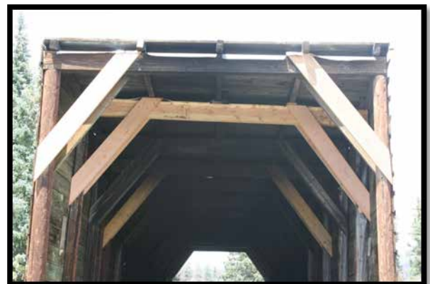
Repairs to the roof have been made and new support bracing has been installed
