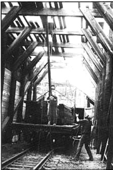
At the Cumbres snowshed, a block and tackle was used to raise decking material from the flat car to the roof. July 1993. Photograph by Terri Shaw.
