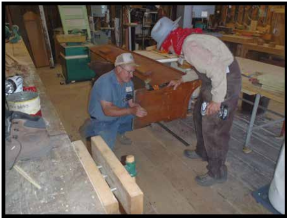
Bob Reib and TL Jim Hickman repair a bench for the Railroad. It is placed on the east side of the Chama Depot and is actually a donated church pew.
