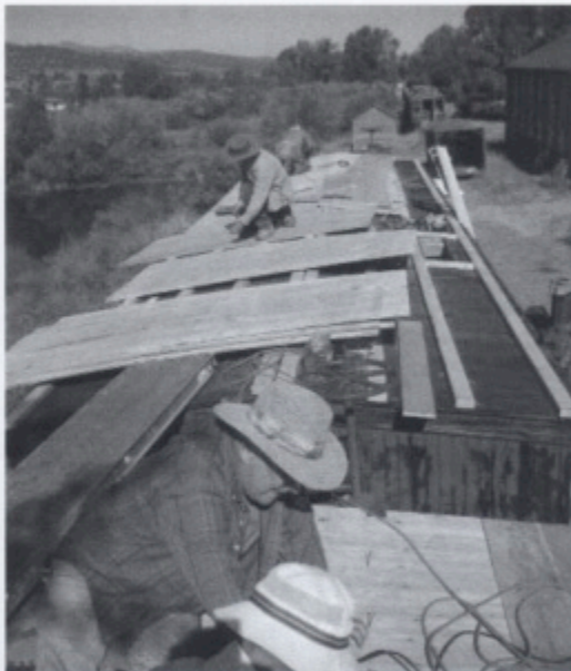
(Front to back) Roger Breeding, Ronald Schaefer, TL Russ Hanscom and Mac Palmer installing new roofs on the Alder Gulch's rolling stock.
