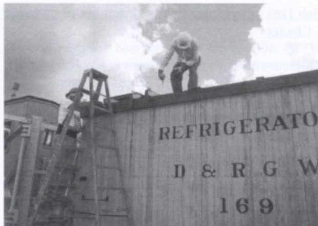
TL Phil Nissen on ladder and Mike Kennedy working on the struts for the ice hatches on the right side/B end of Long Reefer #169.
