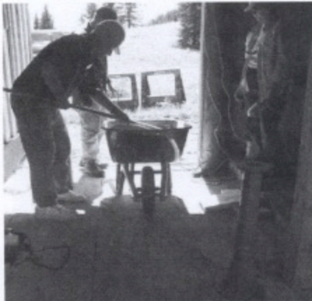
Skip and Dave mix concrete for hand pump base. Laura Kammerer stands ready to assist with placement. Note the cast-iron pump base in the foreground (painted green).
