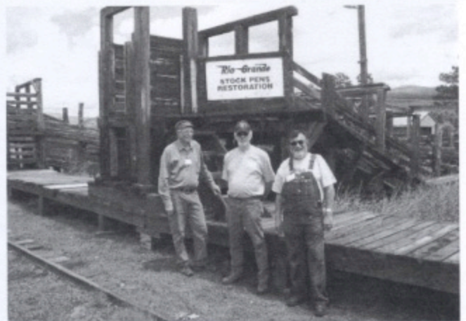
TL Jim Sublett, Len Jones and Bill Jacobs (l-r) on the Chama Sheep Pen Fence Repair team.
