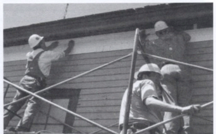
Robert Schoen and Ben Sargent installing new beaded tongue-and-groove siding at trim band, Don Richter assisting.
