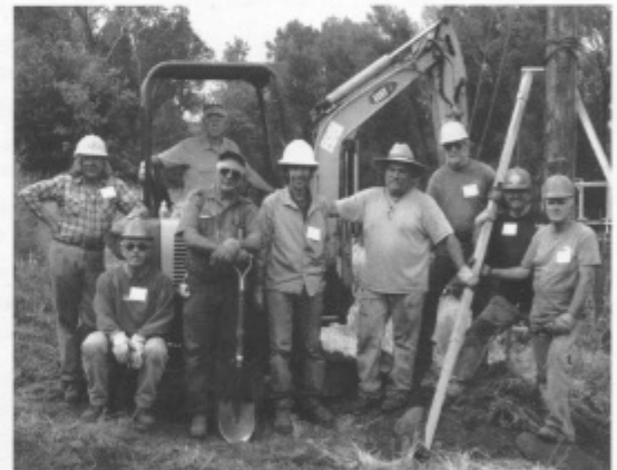
The telegraph pole team has just completed another of the nineteen poles that it placed during Sessions D and F. From left to right are: Wayne Huddleston, Richard Dick, Ron Horejsi, Chris Trunk, John Cole, Larry Woods, Paul Davenport, and Sam Badgett. Bob Hawkins is seated on the excavator. (Jim Galli)
