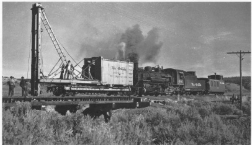
Pile driver OB working on bridge near Amargo, New Mexico on November 18, 1949. From the Denver Public Library Richardson Collection. R.W. Richardson photograph.
