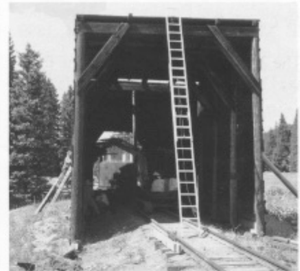
Ron Horejsi is on the outside of the Cumbres snow shed driving nails through the outside wall into the new support beam on the inside. On the inside of the snow shed John Cole and Chris Jensen drive spikes into the base of the same support beam. (Marty Gonzalez)
