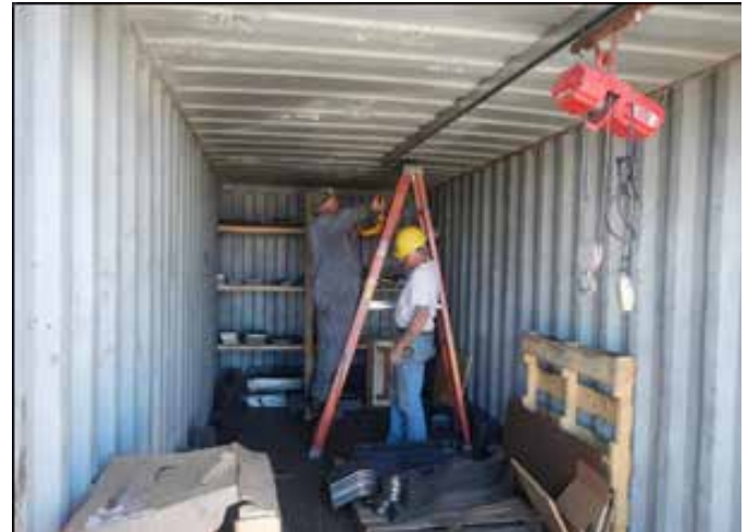
Marshall Smith (on ladder) and Russ Hanscom are installing shelving and a tracked electric hoist which will greatly enhance the utility of the container!
